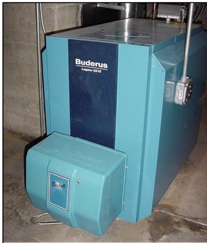
Buderus 'Logano' G215 Heating System with Becket Burner
