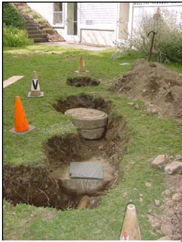
Re-discovered septic system showing outlet, center, inlet access ports (foreground to background) .
