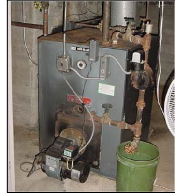
Church heating system installed in 1987. Note the soot buildup around burner.
